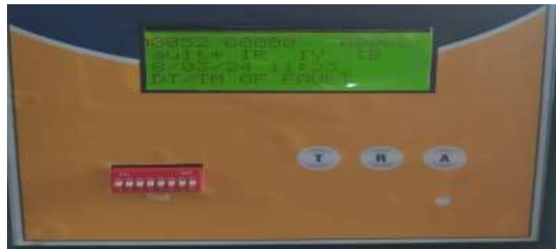
Fig.6: Show last fault data
